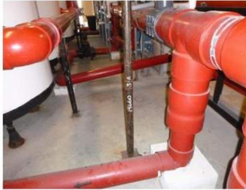
Image 39: Mechanical Room Piping with Concrete Thrust Blocks
