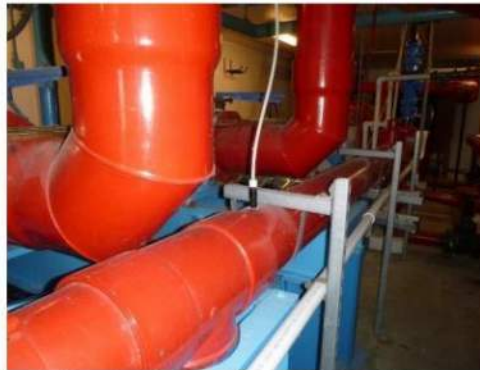
Image 72: Chemical Injection Tap
