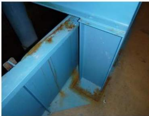
Image 63: Corrosion at Coated Steel Surge Tank
