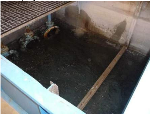
Wave pool surge pit
