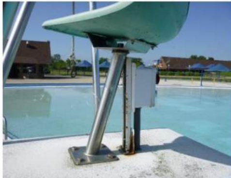
Image 30: Wave Pool Emergency Stop
