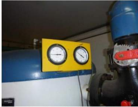
Image 53: Filter Gauge Panel
