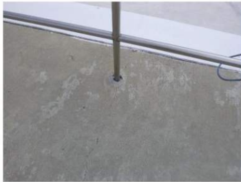
Image 36: Hairline Cracking at Railing Anchor
