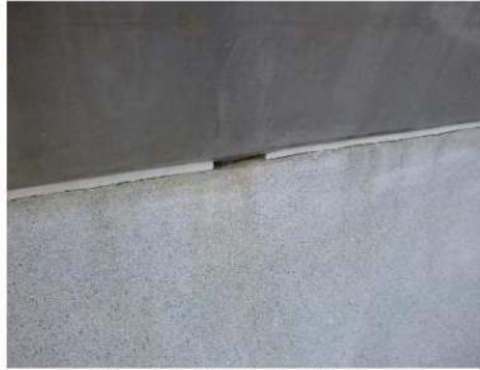
Image 18: Deterioration of Sealant below the Stainless Steel Gutter
