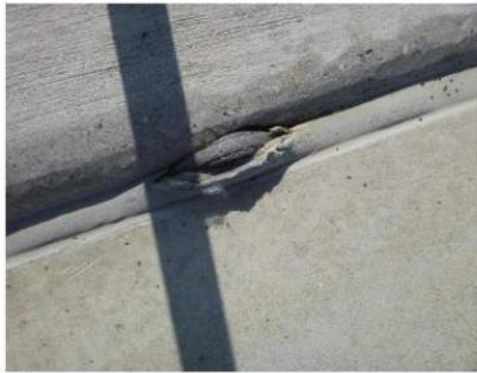
Image 34: Deteriorating Deck Sealant and Exposed Joint Backing
