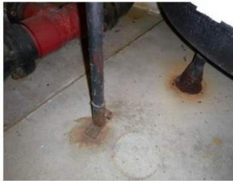
Image 50: Corrosion at Filter Support Leg
