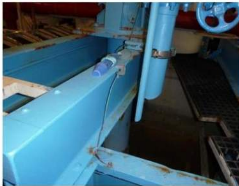
Image 65: Make-up Water Fill at Surge Tank
