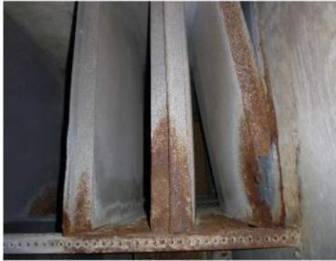
Image 82: Corroded Baffles in Equipment Room
