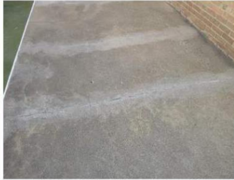
Image 33: Deck Cracking at Wave Caissons
