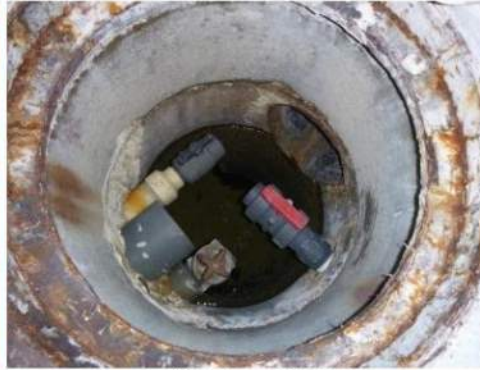
Image 40: Waste Pit Valves
