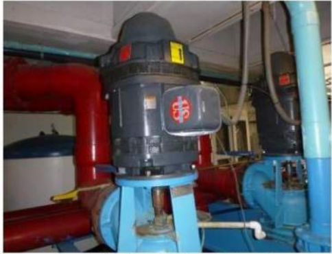
Image 55: Vertical Recirculation Pump
