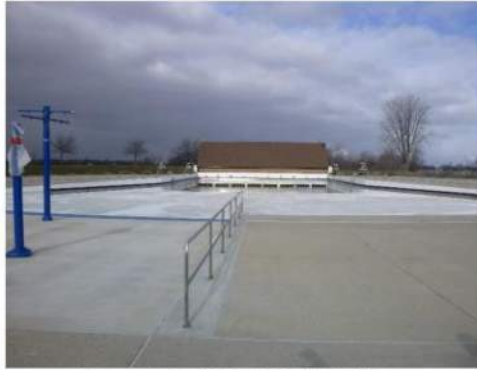
Image 24: Splash Pad Railing
