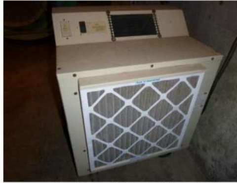
Image 81: Dehumidifier for Wave Pool Equipment Space
