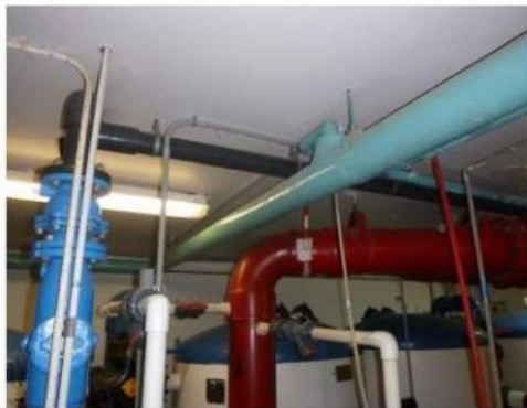
Image 73: Chlorinator Side Stream Taps
