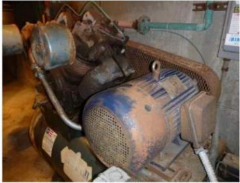
Image 80: Corroded Wave System Air Compressor
