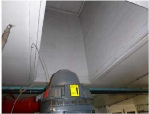
Image 57: Overhead Access for Servicing Recirculation Pumps
