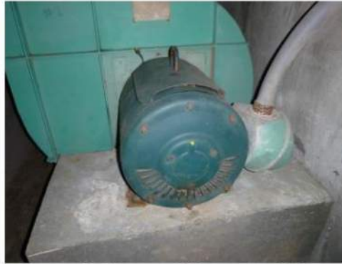
Image 83: Motor and Unsupported Fan
