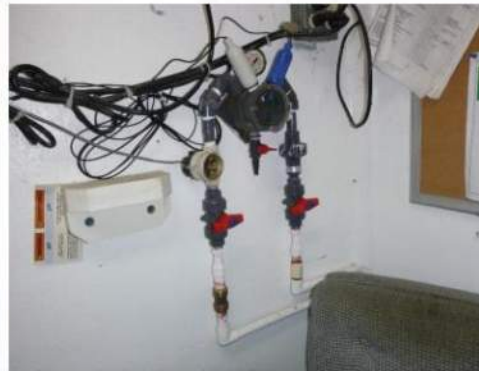
Image 76: Chemical Controller Wiring & Sample Cell
