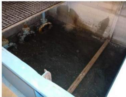
Image 66: Surge Tank During Normal Operation
