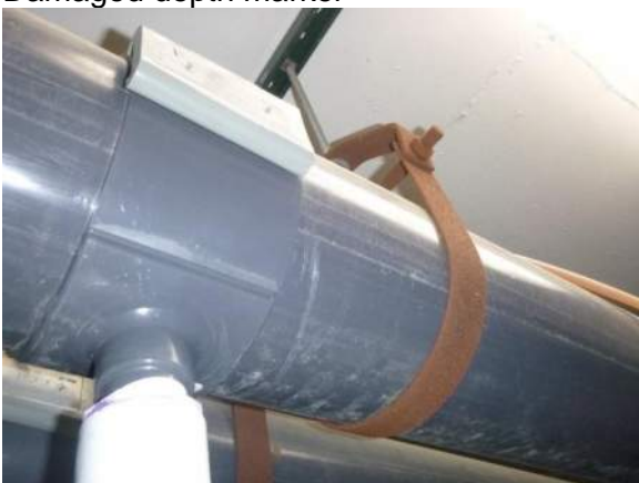
Corroded pipe hanger
