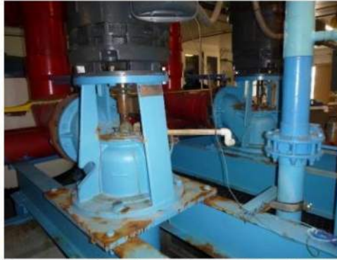
Image 56: Corrosion at Recirculation Pump Base and Frame
