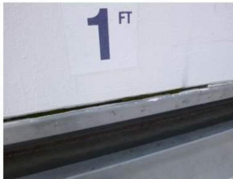
Image 16: Deterioration of Sealant Above Gutter and Concrete
