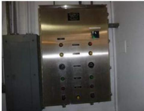
Image 60: Recirculation Pump Starter Panel
