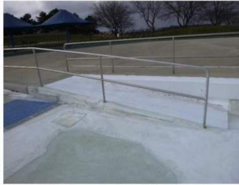
Image 21: Noncompliant ADA Ramp Entry
