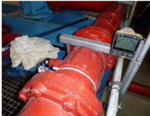
Image 43: Digital Flow Meter Display & Sensor
