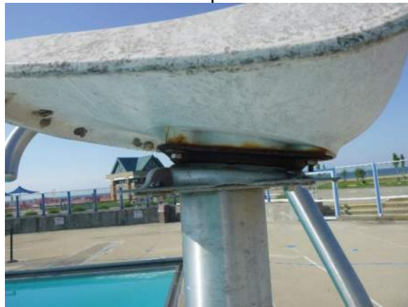
Corroded lifeguard chair seat
