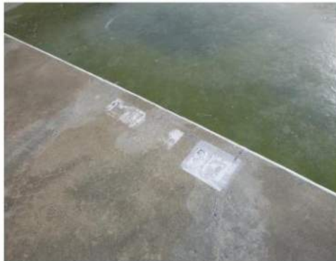
Image 28: Faded Painted Deck Markings
